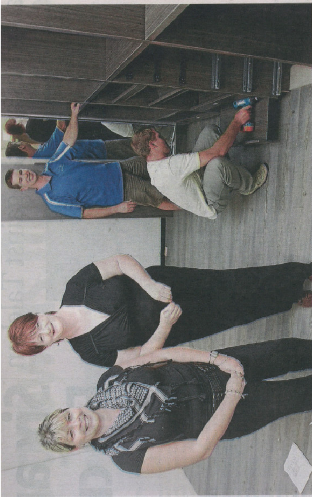
New look: Pridex Kitchens and Innovative Interiors Palmerston North franchise holder Rosie Davey-Hicks, centre, with design consultant Lyn Hesketh as a wardrobe showroom is installed by Dave Harris and Ryan Blinkhorne, bottom.
